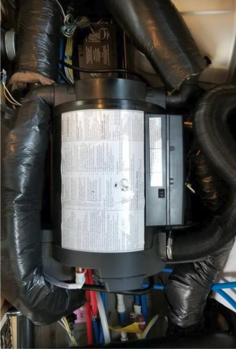
Exposed Truma. Cover is to the right side in this photo
